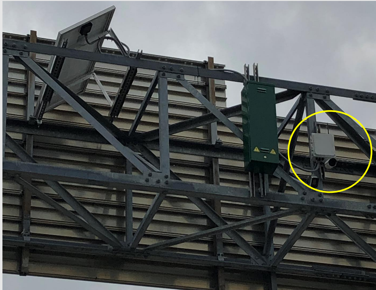
Complex Radar w/video, LED signs and notification (TraffiCalm System)
